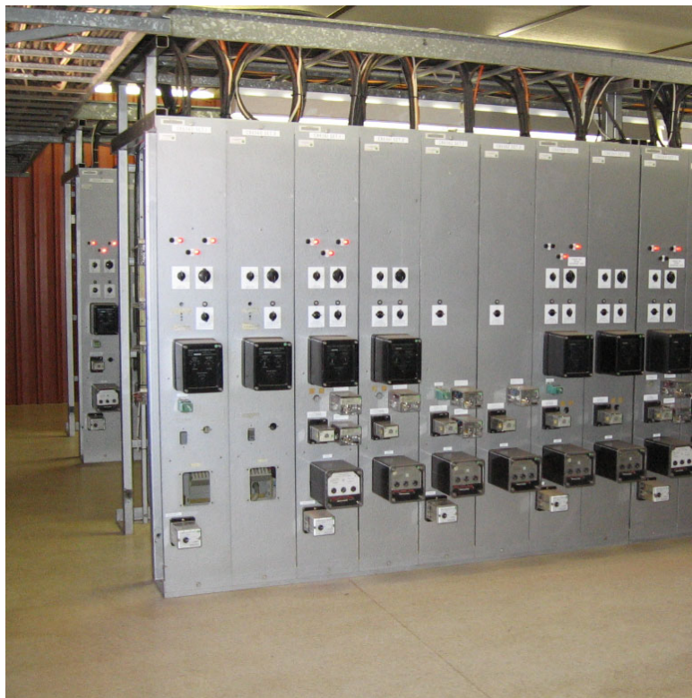
Figure 1 - Protection relays at Davenport substation
