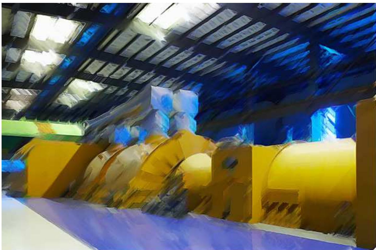
Newport power plant turbine hall
